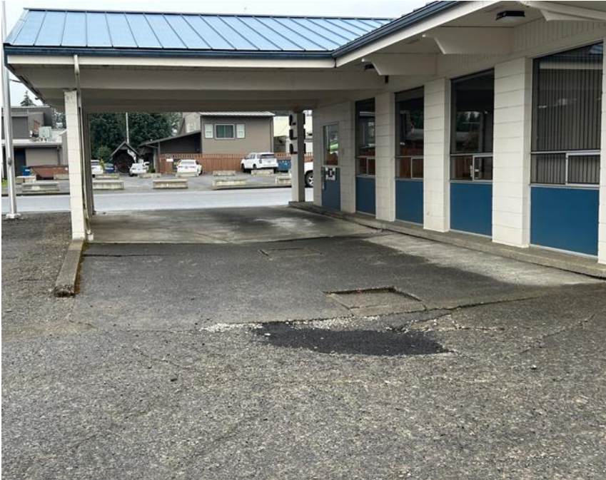
A photo of the Forks parking lot condition (BU 318)
