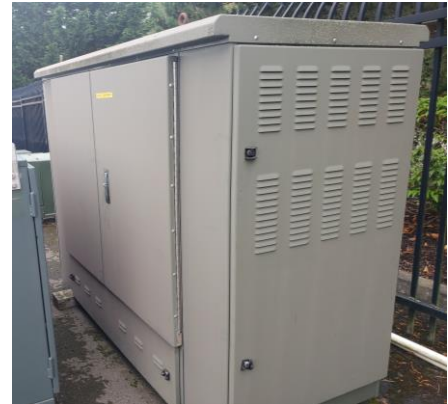
BU 522 Fiber cabinet before installation at Lairds Corner Substation
